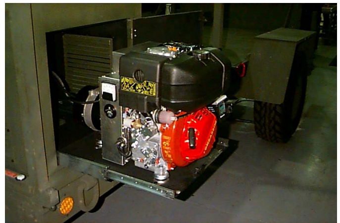
Figure 3-1 - Engine and Generator Location
