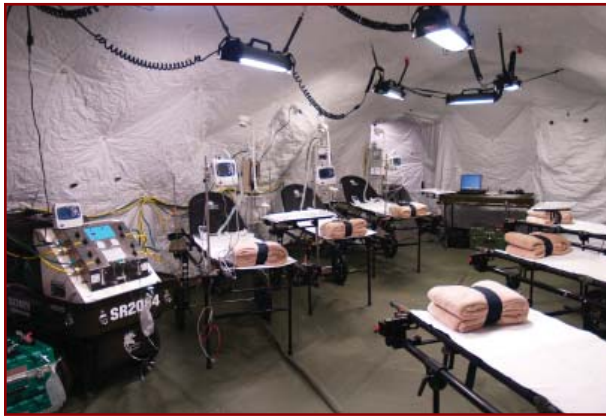
DRASH generators allow medical equipment to run independent of any external power sources.
